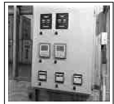
Figure 6. Analyzer Panel at the Artistic Facility
